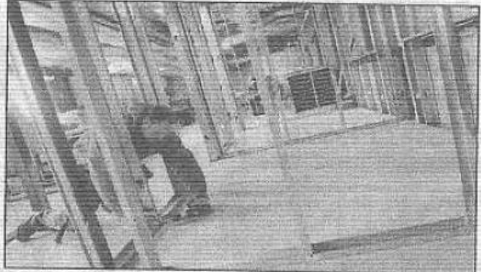
Derek Shibles of Goyette Construction works on the site of the future Wellness Center at the Douglas House in Lexington. STAFF PHOTO BY MATTHEW MODOONO
